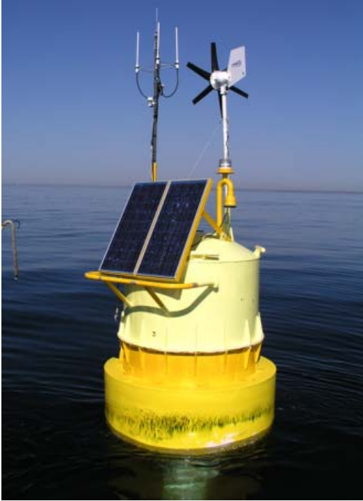
UNH – Open Ocean aquaculture demonstration project. Quarter ton feed buoy with solar and wind charged banks of 120 ah batteries 24 volt batteries.
