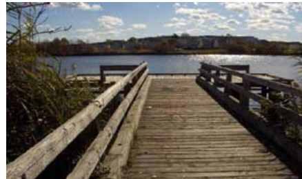
Restore Dock: The existing dock may be repaired. Re-installing benches, adding a railing and signage enhances the users' experience and draws visitors to boat and fish on the river. 2
